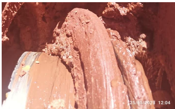
Figure 14. Identification of damaged mancal cover and excess contaminant.
